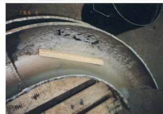
Figure 5-6 – Erosion-corrosion damage due to H 2 Cr in a 10-inch SCR elbow in the outlet of a vacuum heater in a VOU.
